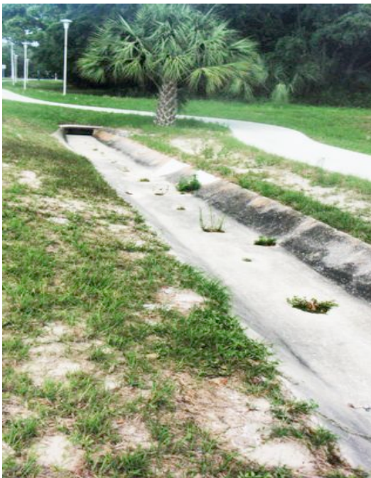
Figure 1 – Conventional drainage channel, Tampa FL, (Putnam, 2010)
